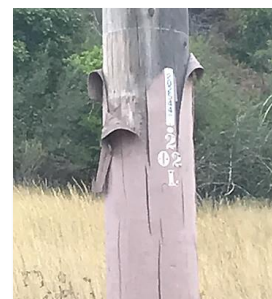
Fire resistant paint tends to fail in about 3-5 years and must be reapplied.
