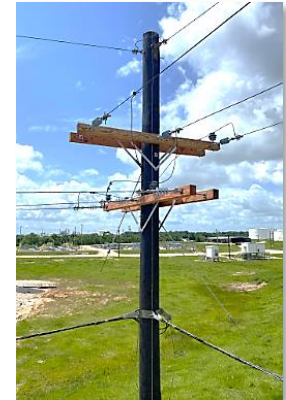
Steel Distribution Pole at a Hard Angle
