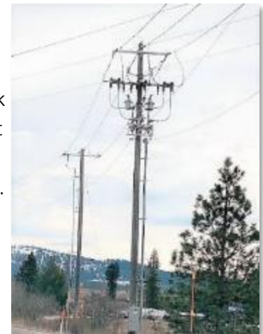
Automation Equipment on a distribution pole in front compared to the pole behind
