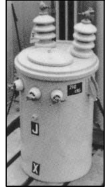
Typical 240Y/480 V, 25 kVA Two-Bushing Transformer
