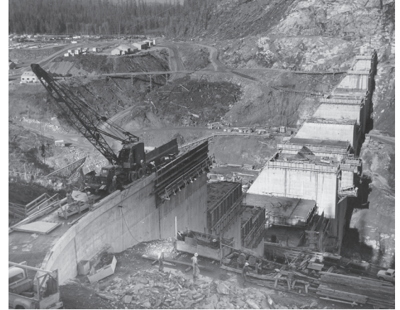
Looking across the entire width of the Baker River canyon (facing downstream), crews work on constructing Upper Baker Dam.
