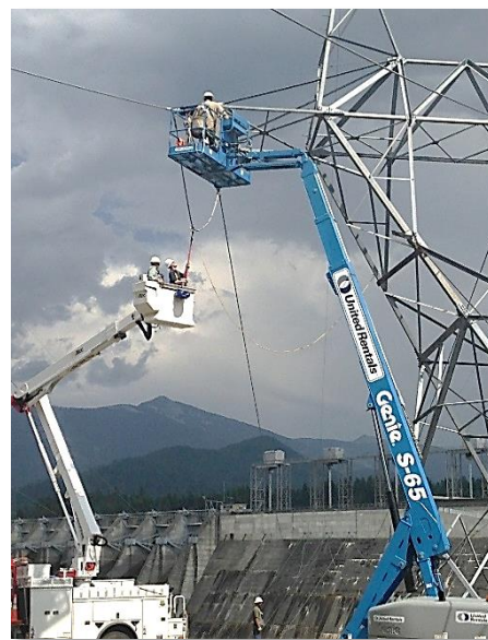
Bucket truck and Genie lift allow crews access to transmission tower at Noxon
