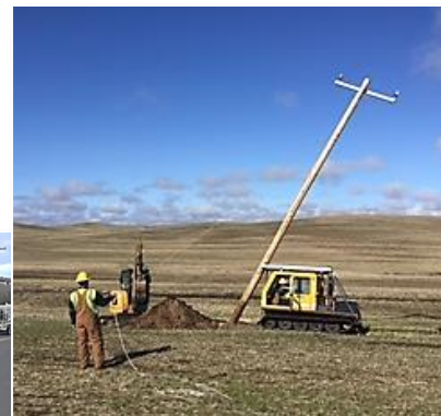
Using a small caterpillar to set a pole on Palouse farmland to minimize field damage
