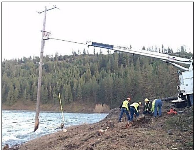
The diversity of conditions across Avista's service territory offers its own challenges. As shown above, crews use a digger derrick to hold up a pole in the river after the riverbank washed out.
