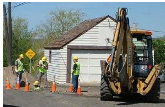
Avista gas crew uses a backhoe to dig up and repair a gas leak in Odessa
