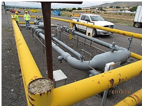
Avista pickup takes a crew to work on Clearwater Paper’s gas system
