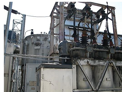
Cabinet Gorge 230 kV Substation breakers
