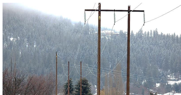
Ninth & Central transmission line
