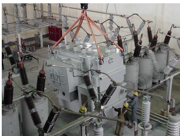
Post Street Sub receives a new transformer to replace one that reached end-of-life
