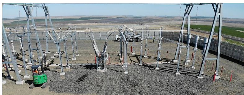
Building the new Neilson Substation to add the Rattlesnake Flat Wind generation to the power grid
