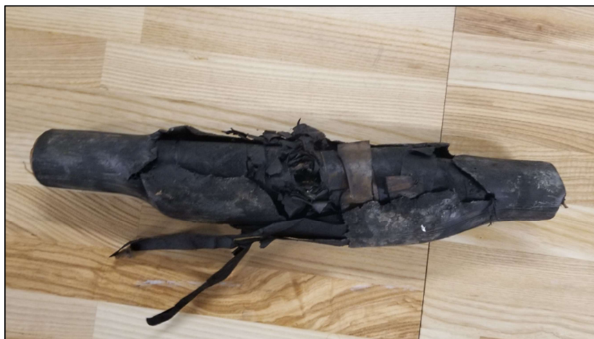
Figure 4: Faulted PILC cabling from peak summer 2018 loading period
