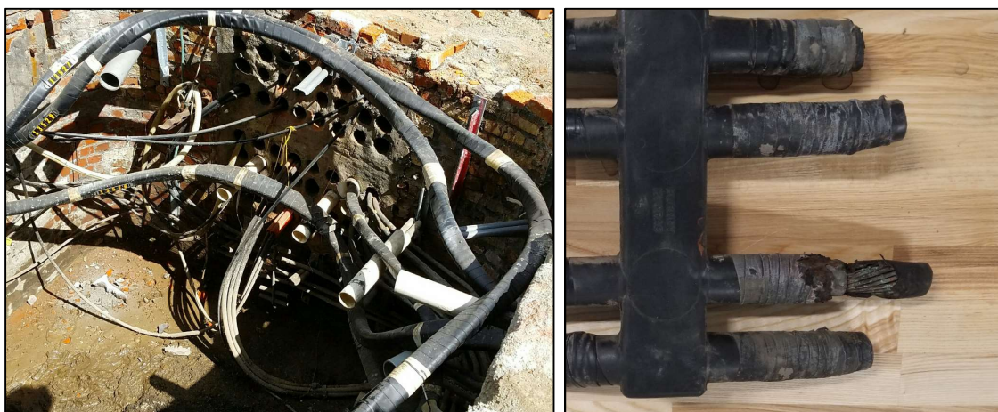
Figure 2: Brick handhole w/assortment of PILC cable / Failed insulation on grid bus (Hotel Ruby Service)
