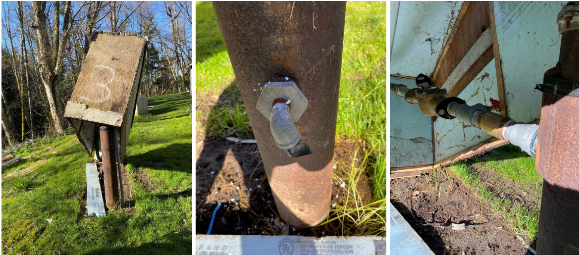
(L) Well #3 (Center) Secondary vent on Well #3 (R) Source meter and sample tap
