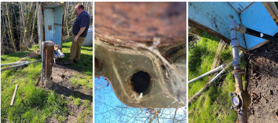
(L) Well #2 (Center) Screened vent on Well #2 (R) Source meter and sample tap
