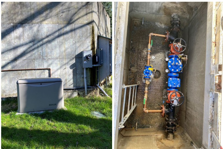
(L) Generator for backup power (R) Newly rebuilt PRV in distribution
