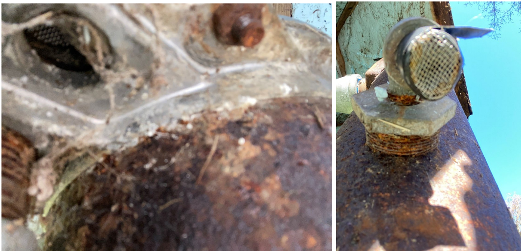
(L) & (R) Screened vents on Well #3
