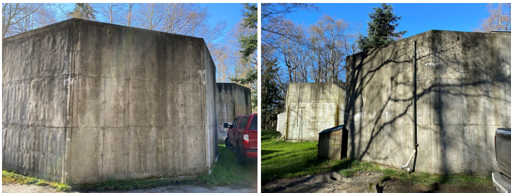
(L) & (R) Existing reservoirs – soon to be demolished once the new tank is finished and online
