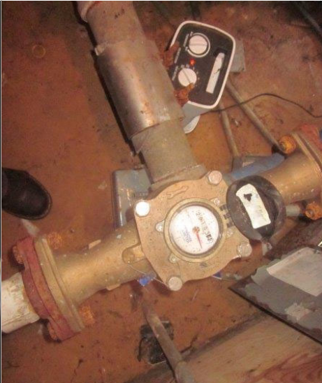
SO1 water meter
