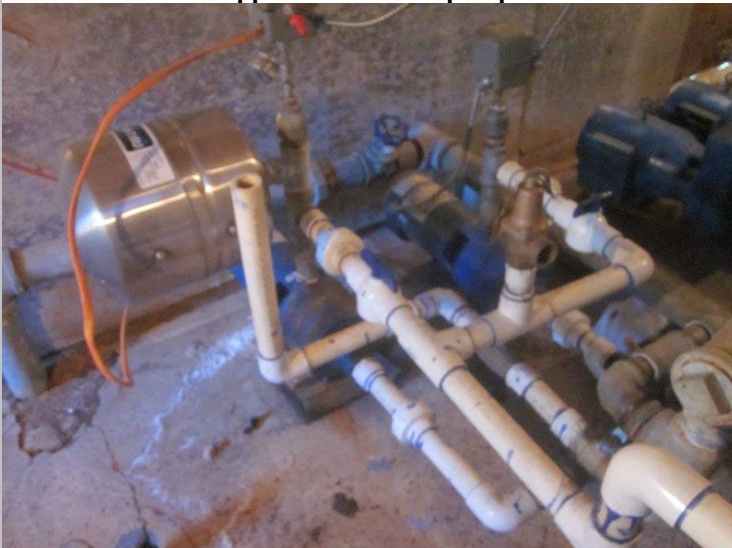
Upper zone booster pumps
