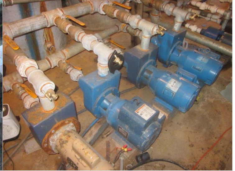
Lower zone booster pumps
