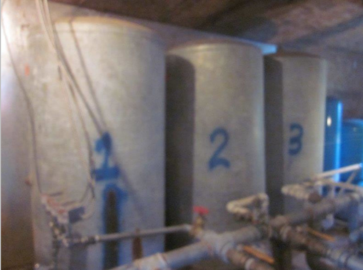
Lower zone pressure tanks
