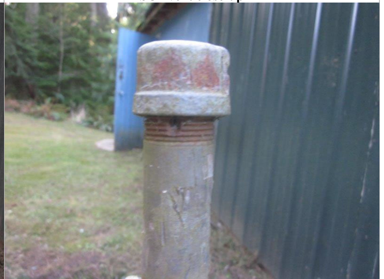
SO2 vent close-up
