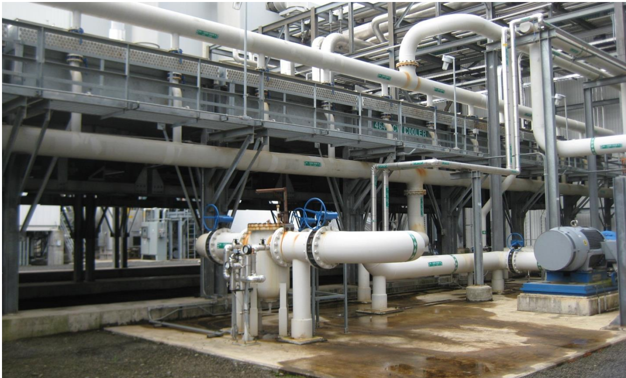
Figure 4: Closed cooling water system with cooler on the left and one of the two 550 HP pumps on the right
