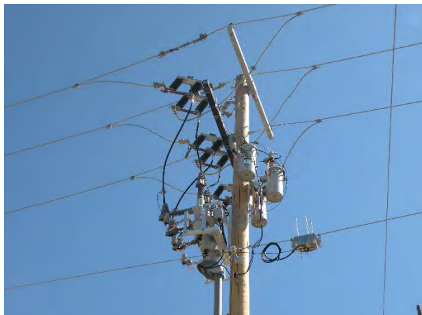
Distribution midline reclosers will play an important role in Avista Next Generation Dry Land Mode program. The ability to quickly detect and de-energize circuits is paramount to reducing fire ignition events.
