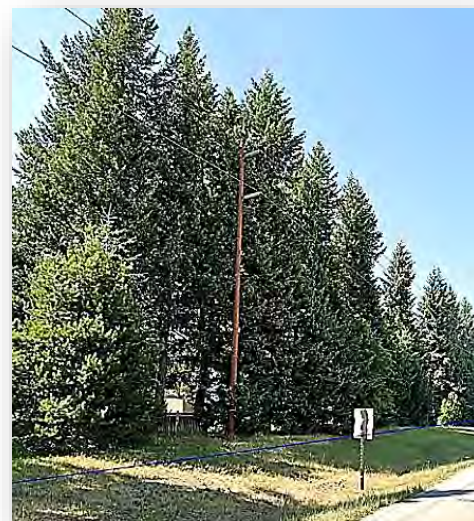
CDA-Rathdrum 115 kV along US Hwy 95
