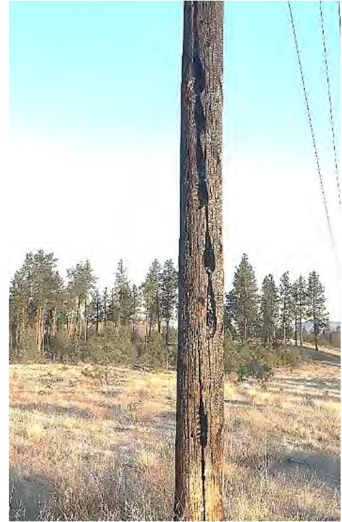
Pole fires generally occur on wood poles with wood crossarms. Since the early 2000's, Avista has adopted fiberglass crossarms as the standard unit. Replacing wood crossarms in elevated fire risk areas is a component of Wildfire Resiliency.
