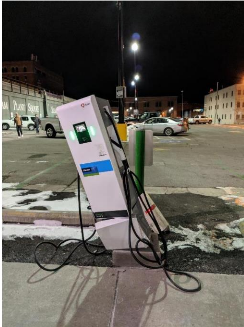
Figure 31. EVSE damage from a vehicle impact
