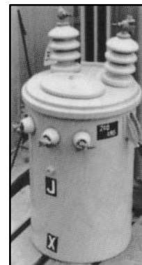
Typical 240Y/480 V, 25 kVA Two-Bushing Transformer
