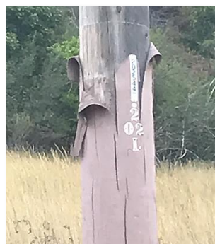
Fire resistant paint tends to fail in about 3-5 years and must be reapplied.
