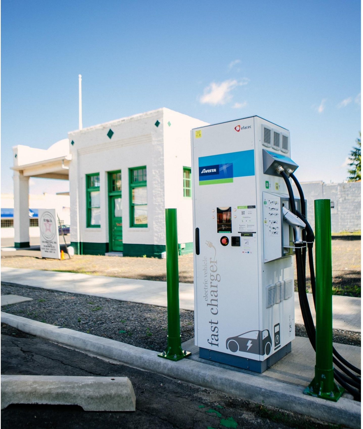
Avista's first DC fast charging site in partnership with the town of Rosalia, Washington (2017)
