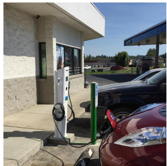
Figure 24: Public EVSE installation
