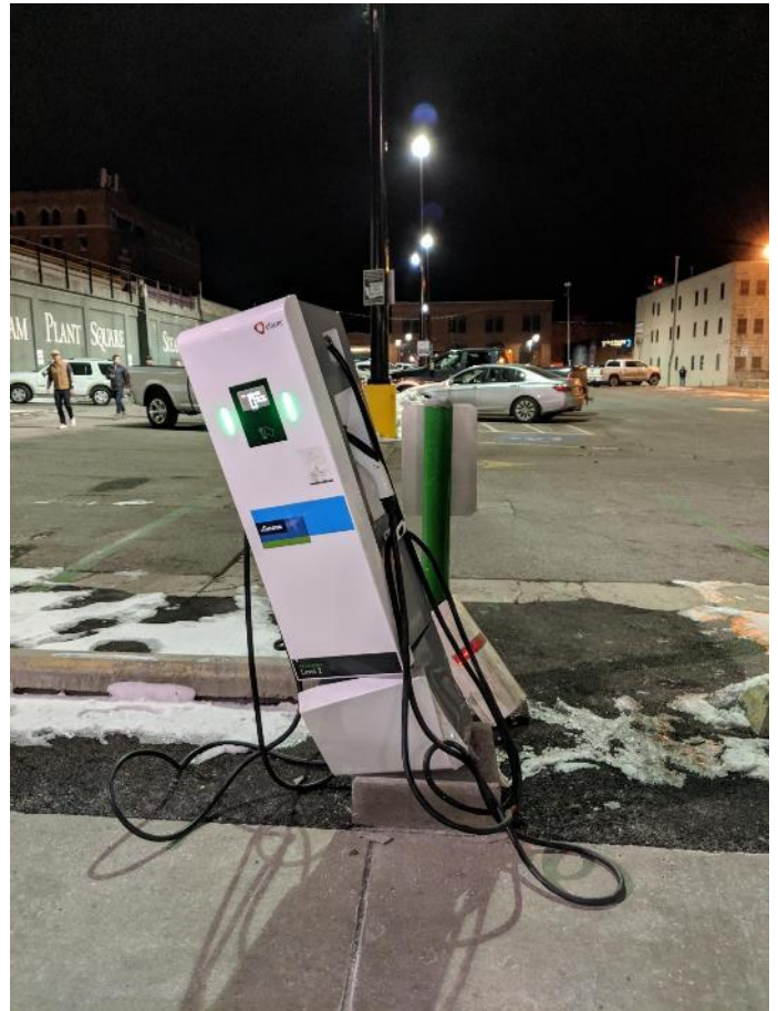
Figure 31. EVSE damage from a vehicle impact
