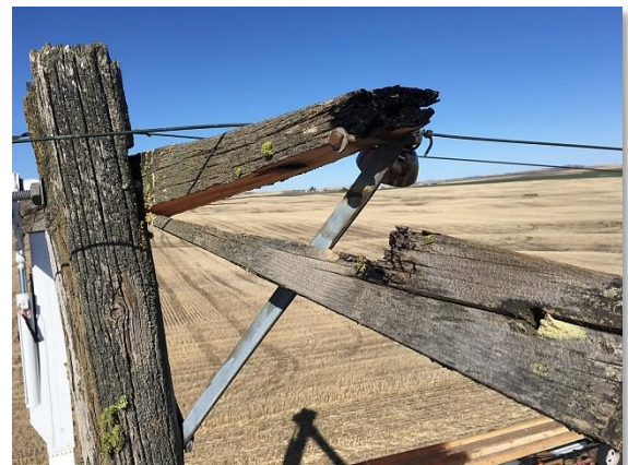
Crossarm tracking fire damage
