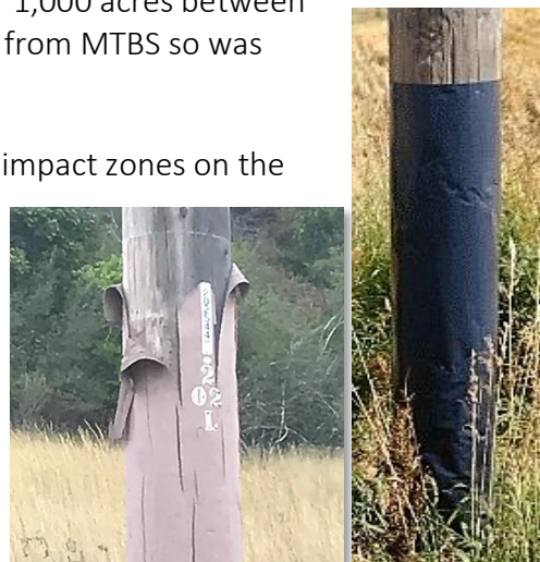
Fire resistant paint tends to crack or peel after about 5 years, so the Company is moving to wire mesh wrap.
