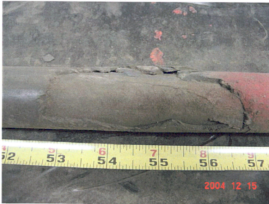
Figure 6. Photograph of Segment 3 showing an area of bare pipe located between the 52.5-inch and 57-inch locations.
