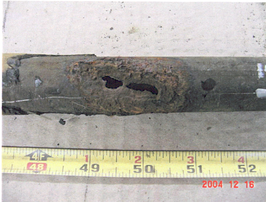
Figure 15. Photograph of Segment 10 after a portion of the coating was removed showing a through wall penetration at the 49-inch location.
