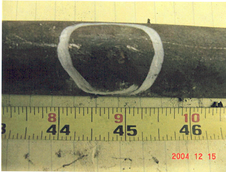
Figure 1. Photograph of Segment 2 after a portion of the coating was removed showing 3 small anomalies at the 45-inch location.
