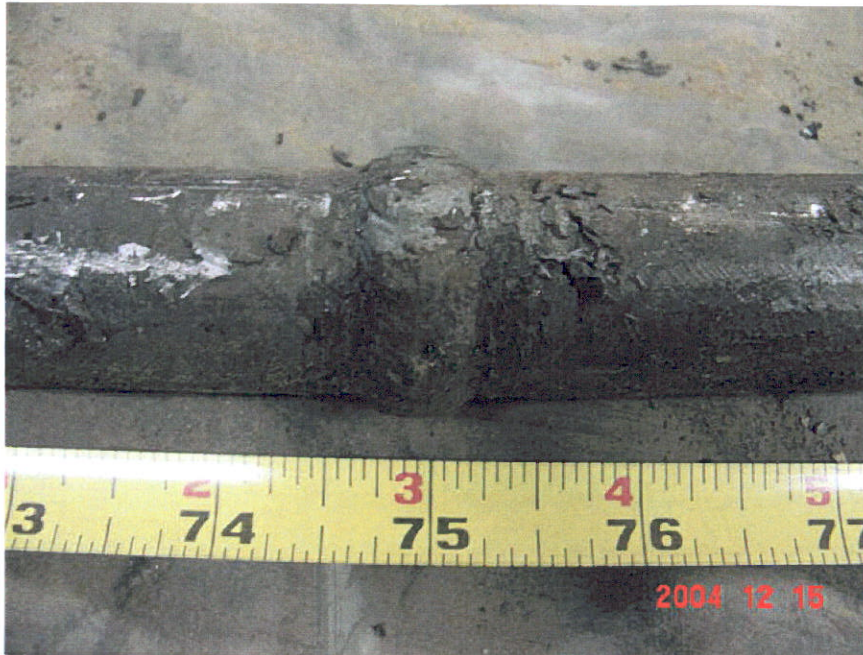
Figure 5. Photograph of Segment 4 after the field applied outer wrap and coating was removed revealing a weld at the 75-inch location.
