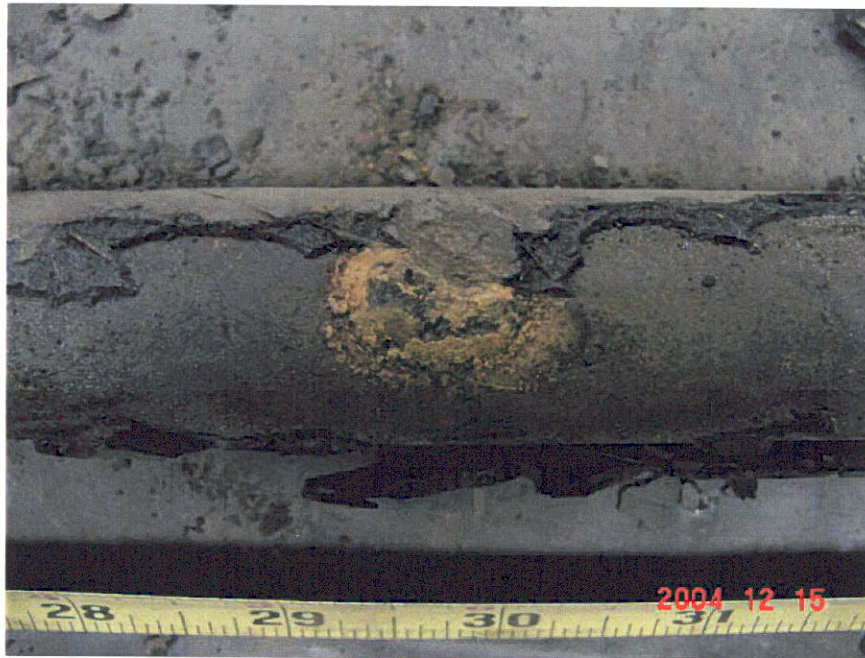
Figure 12. Photograph of Segment 9 after a portion of the coating was removed showing the top of the anomaly at the 29.5-inch location.
