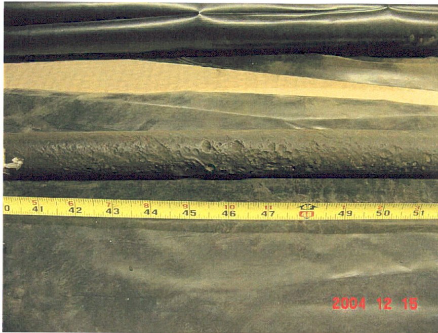
Figure 3. Photograph of Segment 2 showing deformations in the coating from the 40-inch mark to the 53-inch location.
