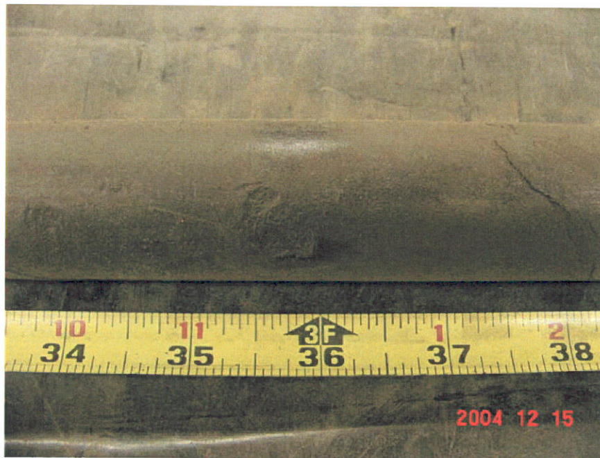
Figure 12. Photograph of Segment 6 showing a coating deformation at the 36-inch location.
