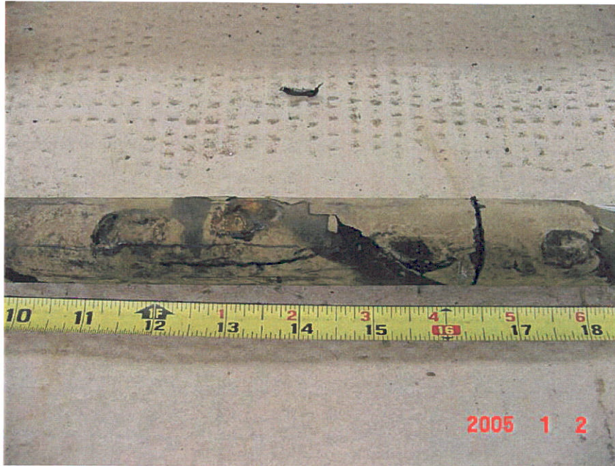
Figure 29. Photograph of Segment 10 showing coating deformations ranging from 0.5 to 2-inches long between the 11 and 24-inch locations.
