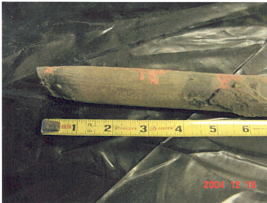
Figure 2. Photograph of Segment 2 showing a crimp at the 0-inch location of the pipe and an area of bare pipe from 0 to 8-inches.
