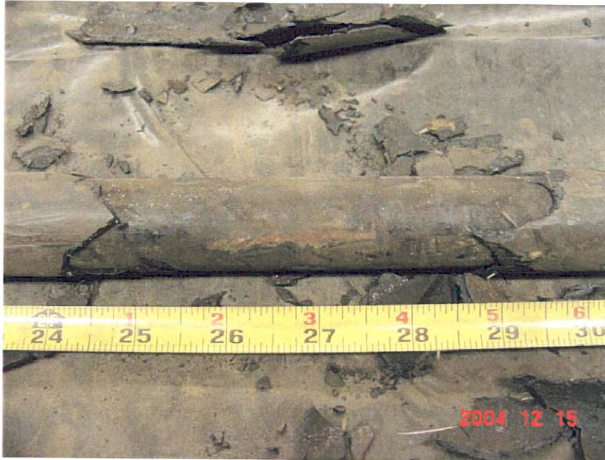
Figure 7. Photograph of Segment 7 after removal of a portion of the coating showing no corrosion under the gouge in the coating to bare pipe that was located at the 26-inch location.
