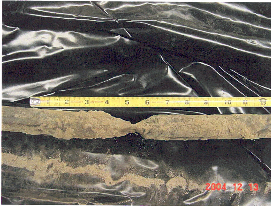
Figure 7. Photograph of unwrapped Segment 2 showing a crimp in the pipe located at 57.5-inches downstream from the end of the cut.
