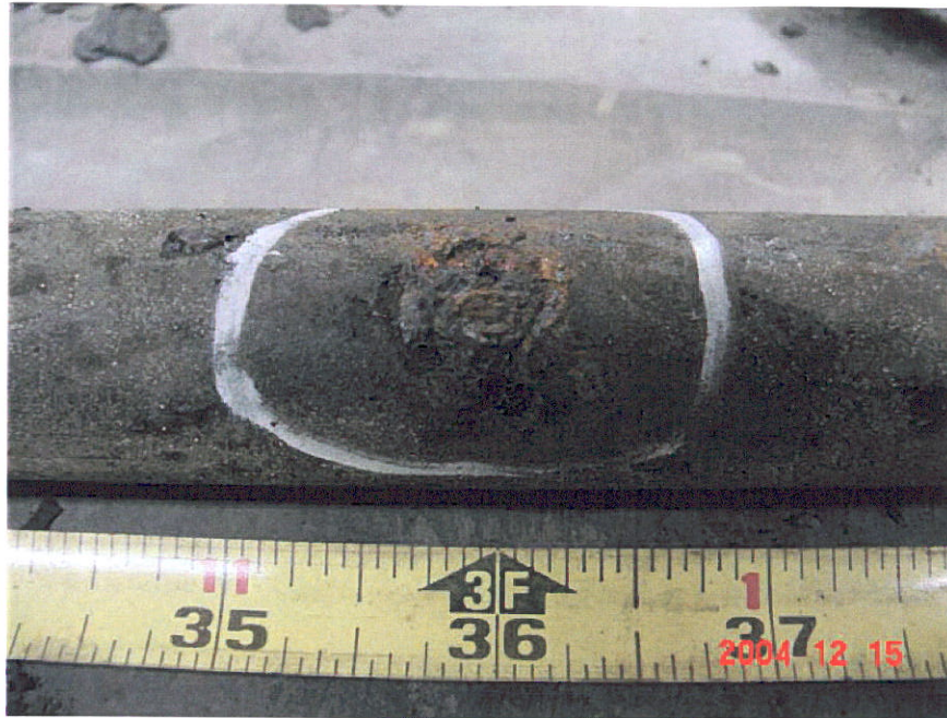
Figure 13. Photograph of Segment 9 after a portion of the coating was removed showing an anomaly at the 36-inch location.
