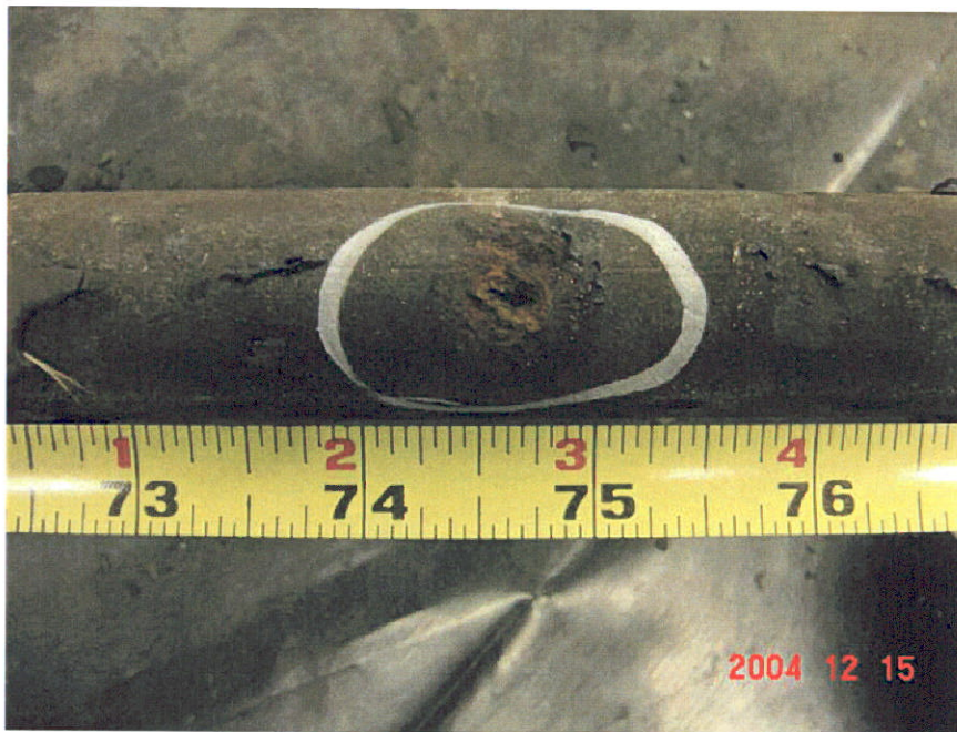
Figure 2. Photograph of the Segment 2 after a portion of the coating was removed showing a 0.25-inch anomaly at the 74.5-inch location.
