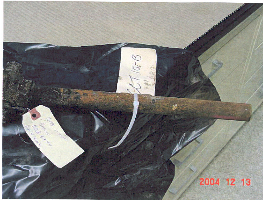
Figure 39. Photograph of unwrapped Segment 10 showing the downstream side of the pipe, CCT 10-B.
