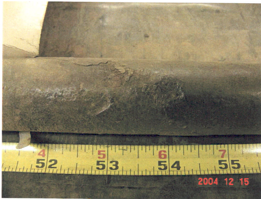
Figure 14. Photograph of Segment 6 showing a coating deformation at the 54-inch location.
