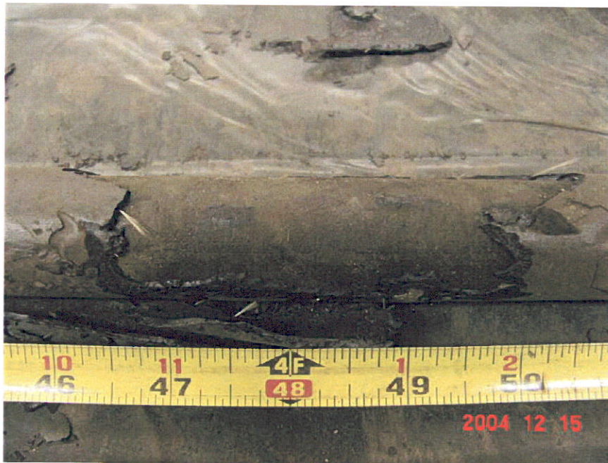
Figure 8. Photograph of Segment 7 after removal of a portion of the coating showing no corrosion in the pipe underneath the coating holiday at the 48-inch location.
