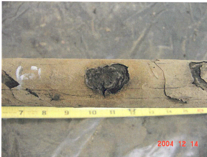
Figure 30. Photograph of Segment 10 showing a 2-inch coating deformation at the 21-inch location.
