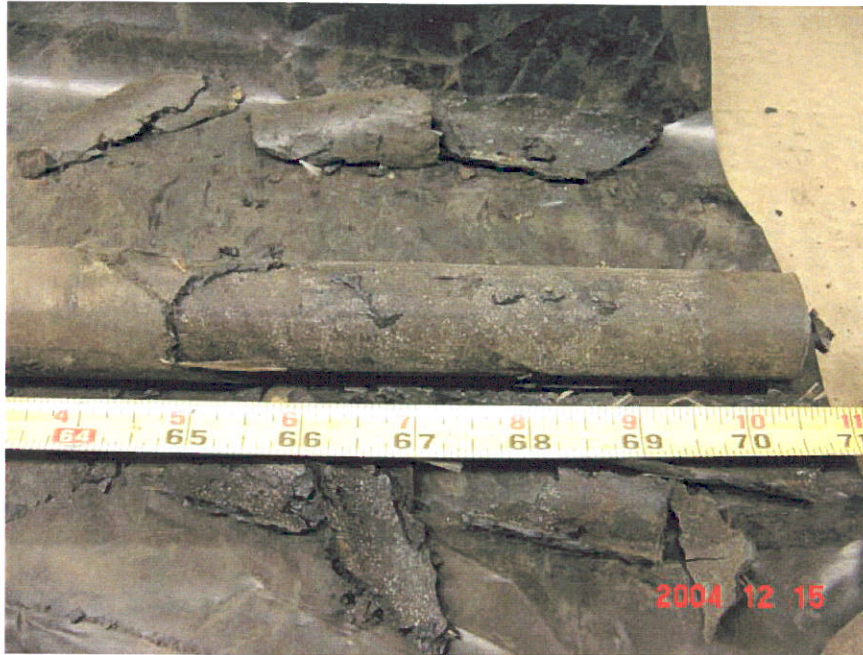
Figure 9. Photograph of Segment 7 after removal of a portion of the coating showing no corrosion underneath the coating holiday that was at the 66-inch location.
