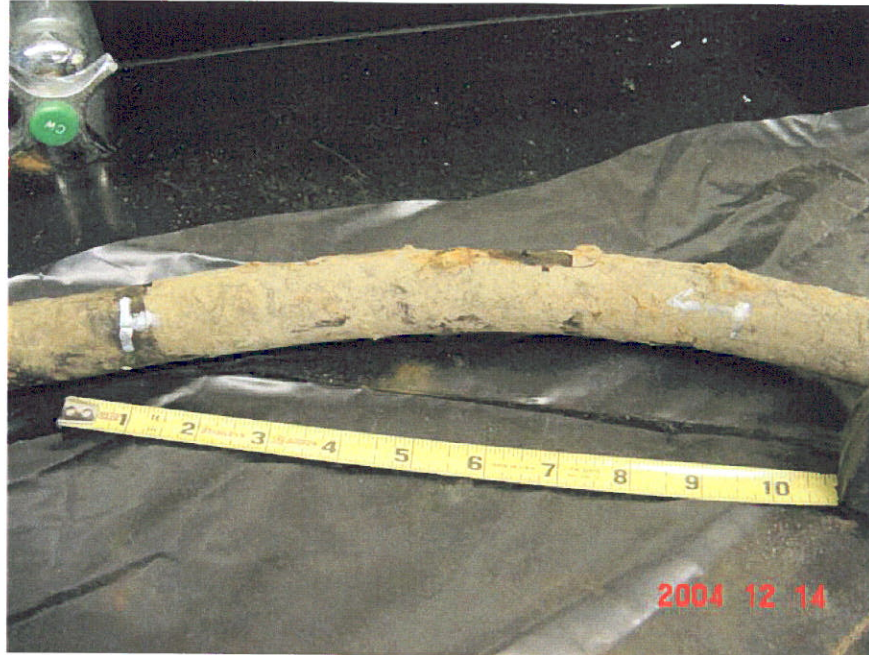
Figure 33. Photograph of Segment 10 showing the bend in the pipe that contained 6 areas of coating deformations on the extrados starting at the 57.75-inch location.
