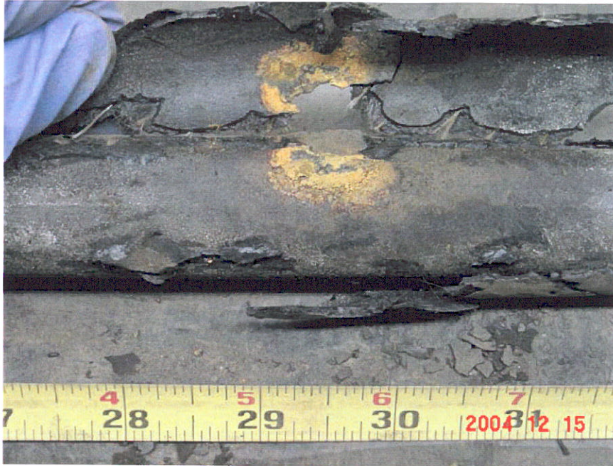
Figure 5. Photograph of Segment 9 showing an anomaly at the 29.5-inch location.
