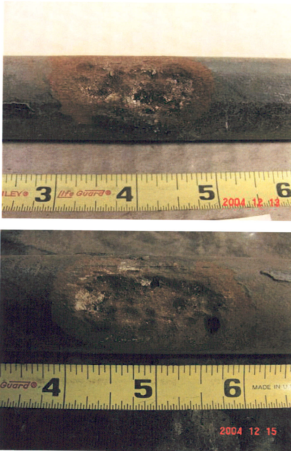
Figure 10. Corrosion site in Segment 1. Top photo shows the surface condition prior to the surface cleaning. Bottom photo shows the surface without the debris.
