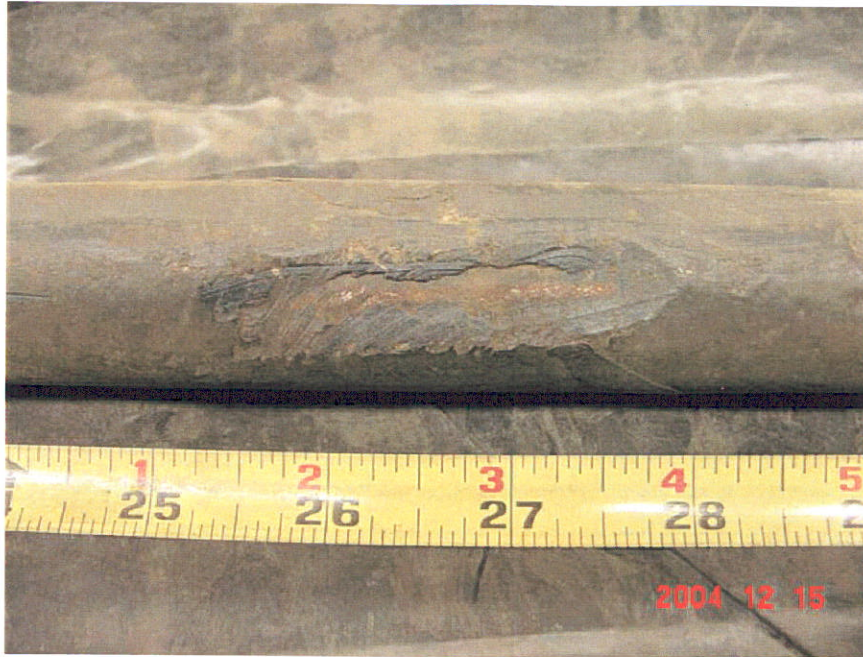
Figure 17. Photograph of Segment 7 showing a gouge in the coating from the 25-inch to 28-inch locations.
