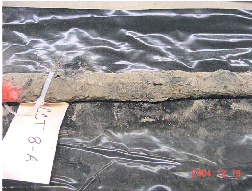
Figure 28. Photograph of unwrapped Segment 8 showing the upstream side of the pipe, CCT 8-A.
