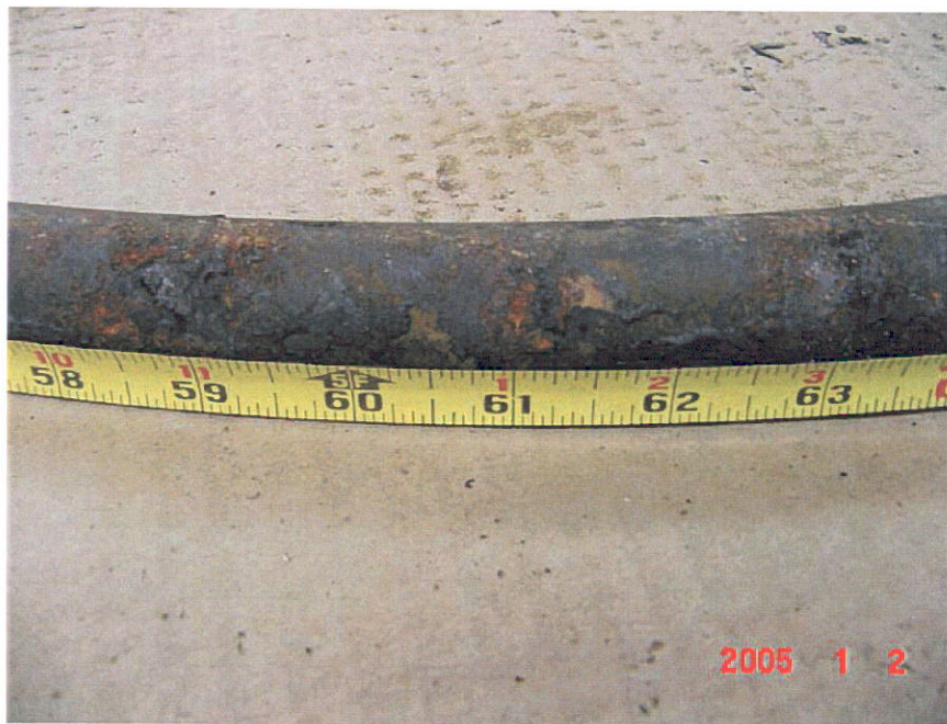
Figure 16. Photograph of Segment 10 after a portion of the coating was removed showing the corrosion colored product that was present on the extrados of the bend in the pipe.
