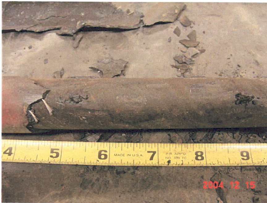
Figure 6. Photograph of Segment 4 after removal of a portion of the coating showing no corrosion underneath the coating holidays at the 6-inch location.
