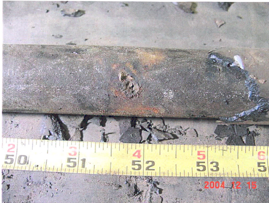
Figure 3. Photograph of Segment 1 showing an anomaly at the 51.75-inch location.
