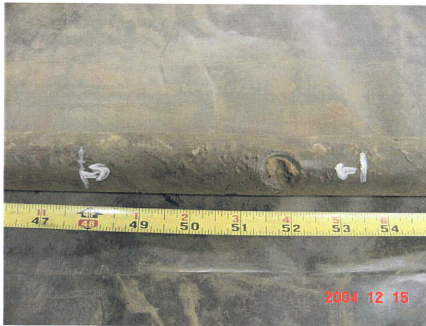
Figure 8. Photograph of Segment 4 showing a coating deformation at the 52-inch location.
