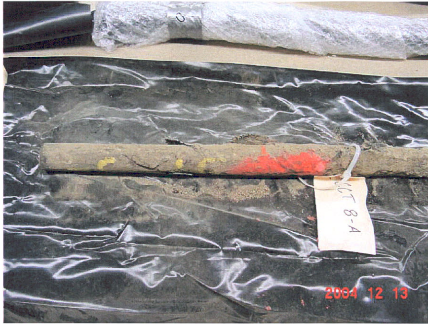
Figure 27. Photograph of unwrapped Segment 8 showing the upstream side of the pipe, CCT 8-A.
