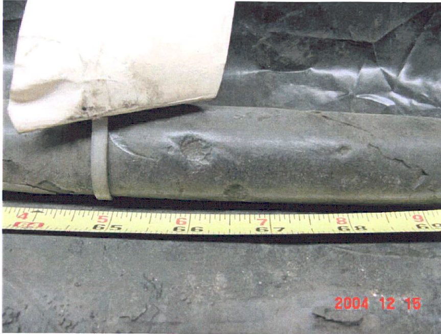
Figure 19. Photograph of Segment 7 showing a deformation in the coating at the 66-inch location.
