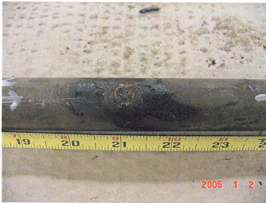
Figure 14. Photograph of Segment 10 after a portion of the coating was removed showing an anomaly at the 21-inch location.
