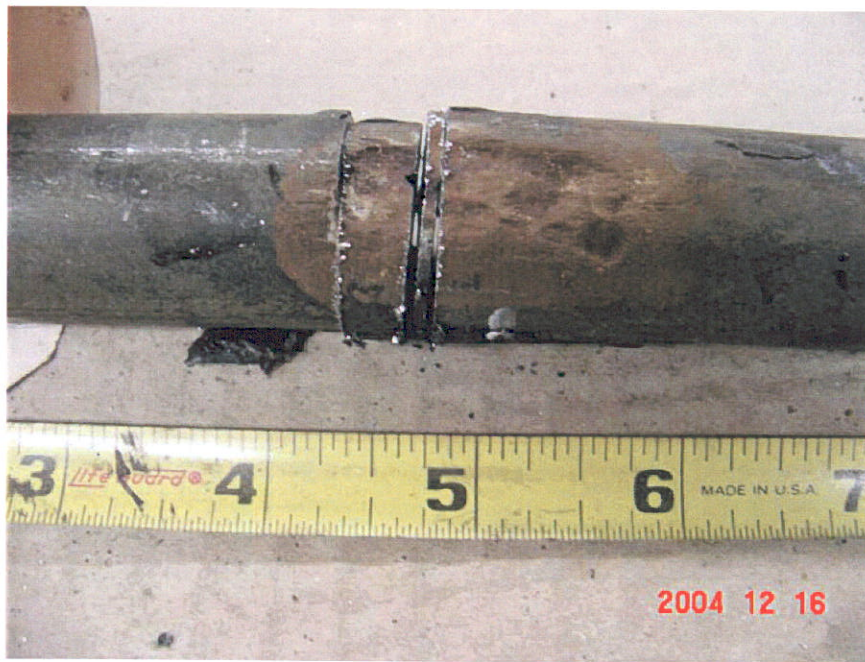
Figure 2. Photograph of Segment 1 showing where Mount 1-B (2 nd piece from left) and Surface 01-C (3 rd piece from left) were cut out of the pipe.
