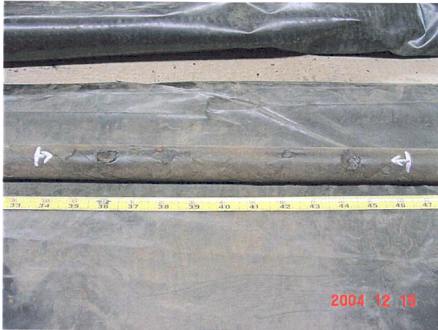
Figure 27. Photograph of Segment 9 showing deformations and dents in the coating between the 34-Inch location and the 46-inch location.
