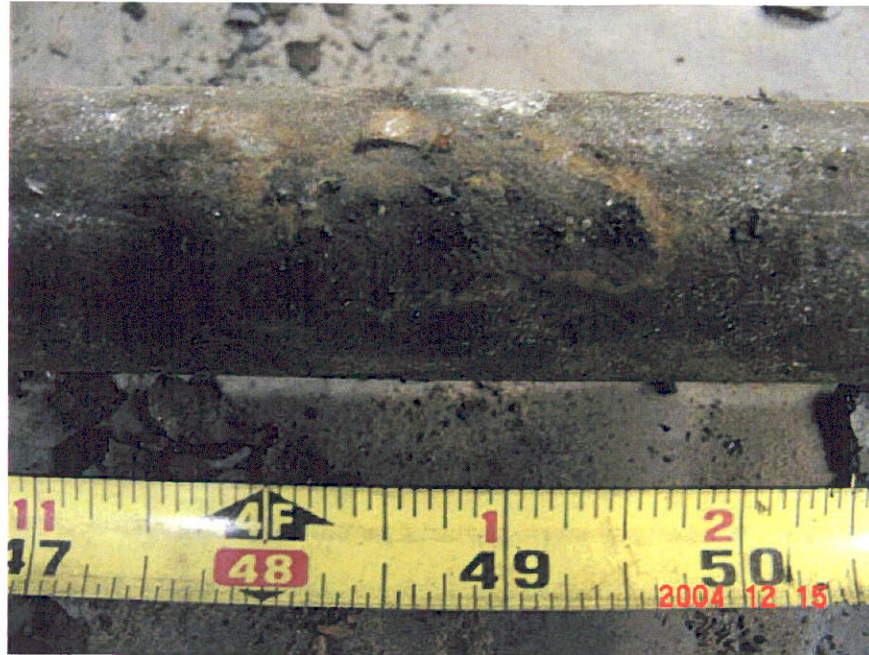
Figure 3. Photograph of Segment 4 after a portion of the coating was removed showing 1.5-inch anomaly area under disbonded coating.
