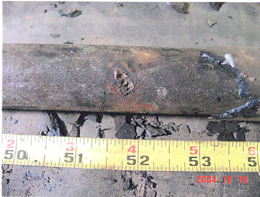
Figure 4. Photograph of Segment 4 after a portion of the coating was removed showing a 0.25-inch anomaly at the 51.75-inch location.
