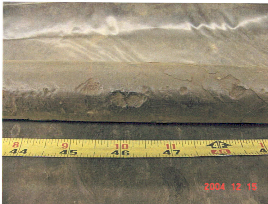
Figure 18. Photograph of Segment 7 showing coating deformations and dents in the coating that extended between the 41.5-inch to 55-inch locations.
