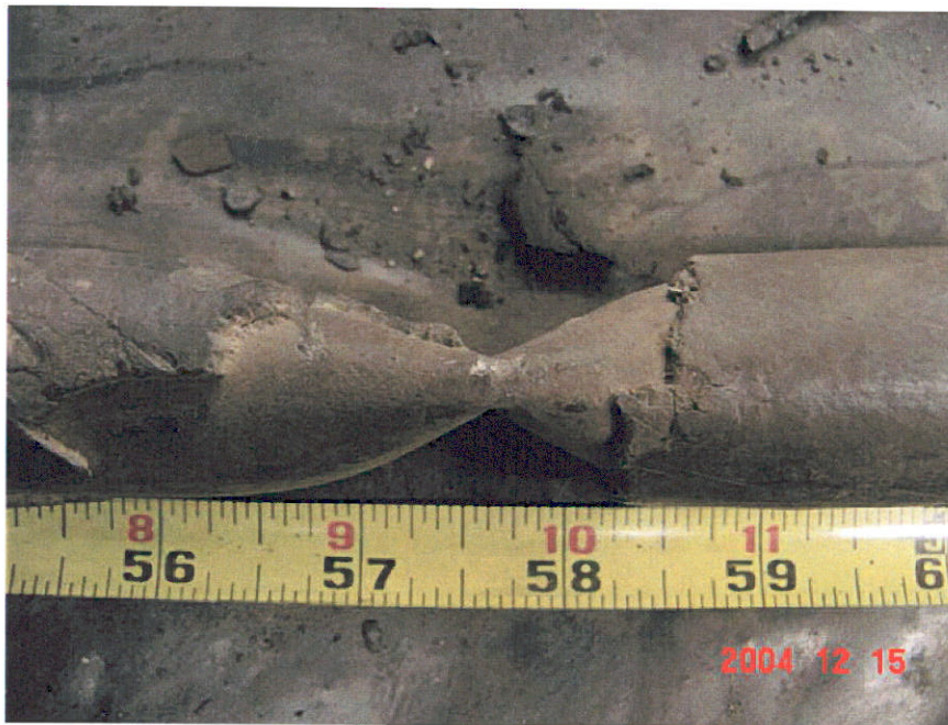
Figure 4. Photograph of Segment 2 showing a crimp in the pipe at the 57.5-inch location.
