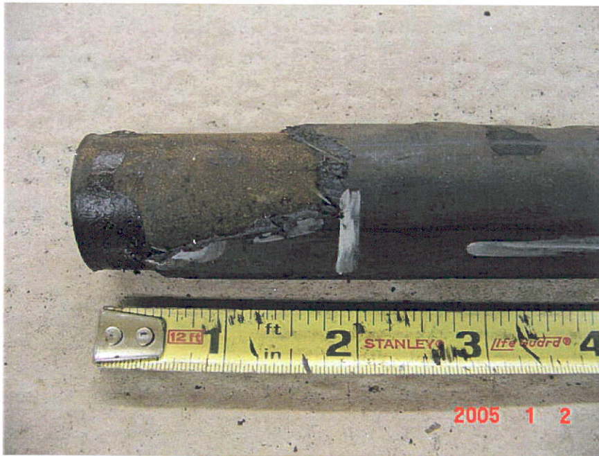
Figure 28. Photograph of Segment 10 showing a 2-inch area of bare pipe at the 0-inch location.
