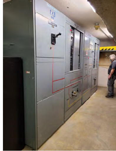
Existing 208/120V Main Switchboard located in basement
