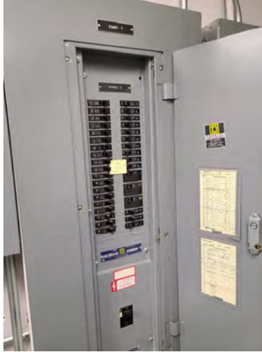
Existing age of Panelboards in Building
