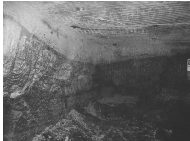
Figure 6. Photograph of a slump feature encountered in the Upper B Seam gate entry development.
