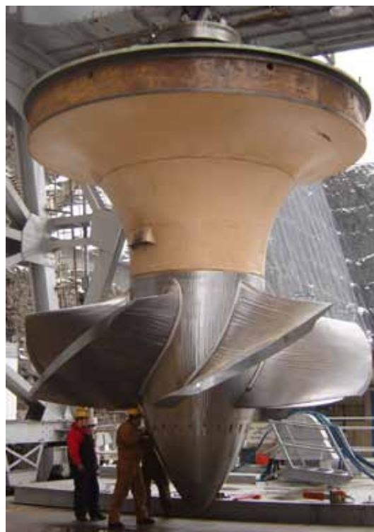
Noxon Rapids turbine upgrade
