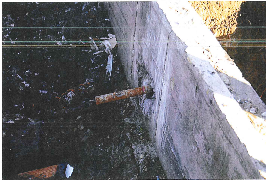
Photo 9: View of the gas fuel pipe entry into crawl space through east foundation wall. The vertical saw cuts in the concrete wall were made after the incident. Photo taken October 18, 2011, by Dennis Ritter, UTC engineer
