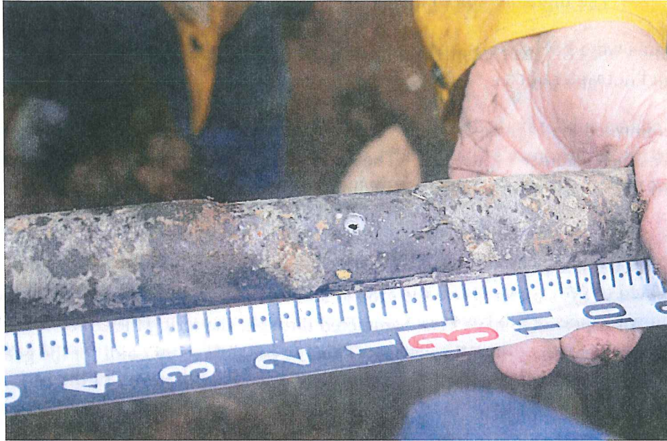
Photo 8: View of the hole in gas service pipe to Inghams' home located on bottom side of the pipe where it crossed over the sewer pipe. Photo taken September 26, 2011, by Al Jones, UTC engineer.
