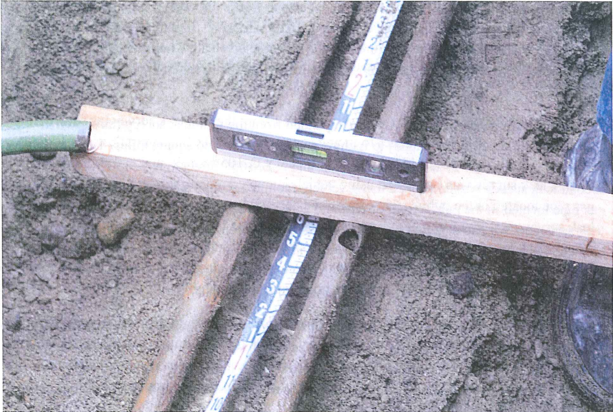
Photo 5: View of service pipe at 1020 N.E. 127 th Street, where the high voltage passed from the abandoned water pipe (rust colored line with a hole) to the gas service pipe (green coated pipe). The damaged gas service pipe had been removed at the time this photo was taken. Photo taken October 20, 2011 by David Cullom, UTC engineer.
