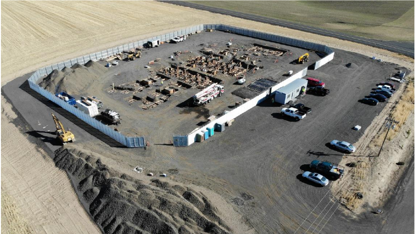
NEILSON SWITCHING STATION – RATTLESNAKE FLAT WIND INTEGRATION
