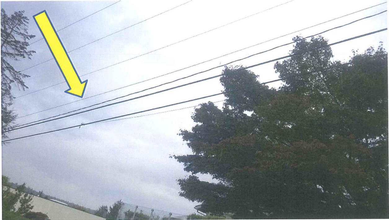
To close to power at mid-span. 30 inch minimum separation required.
