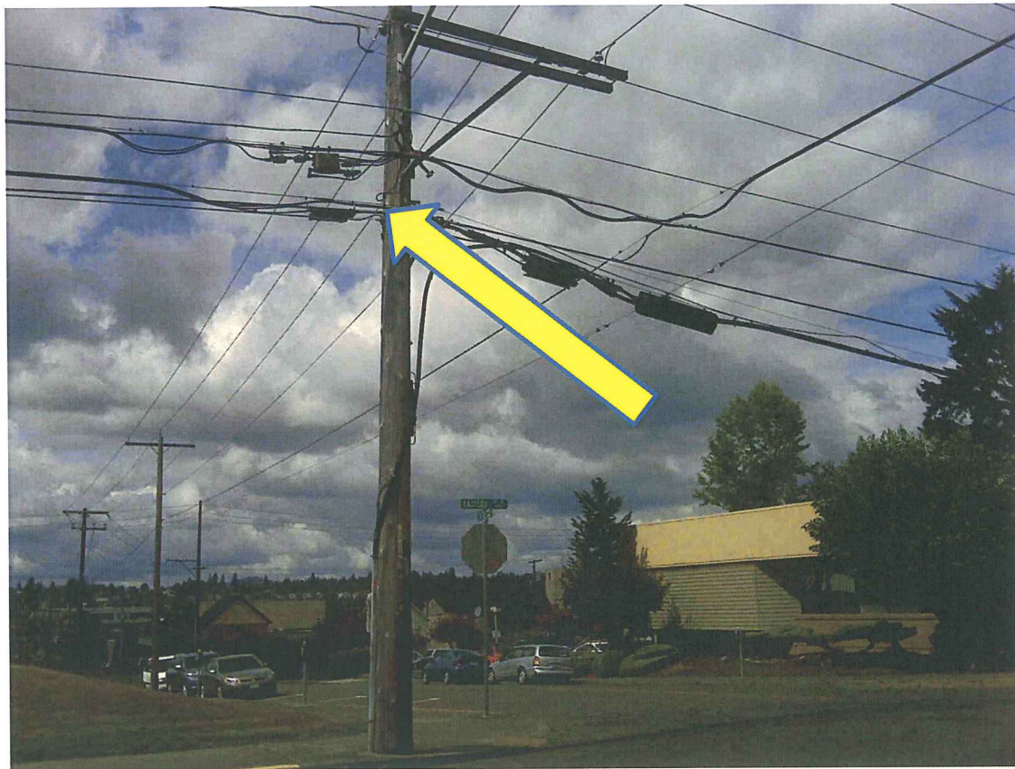
Too close to power. Incorrect build/install.
