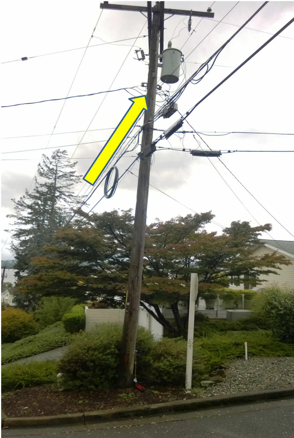
Figure 1: Both communications attachments are too close to power. Lowest power is the bottom of the drip loop. Overlashing had occurred one week prior to this picture being taken.
