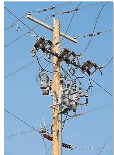
Figure 20. Dry Land Mode Device: Viper Recloser
