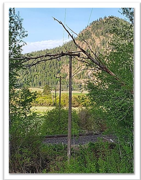
Figure 16. Dead tree falls into powerline
