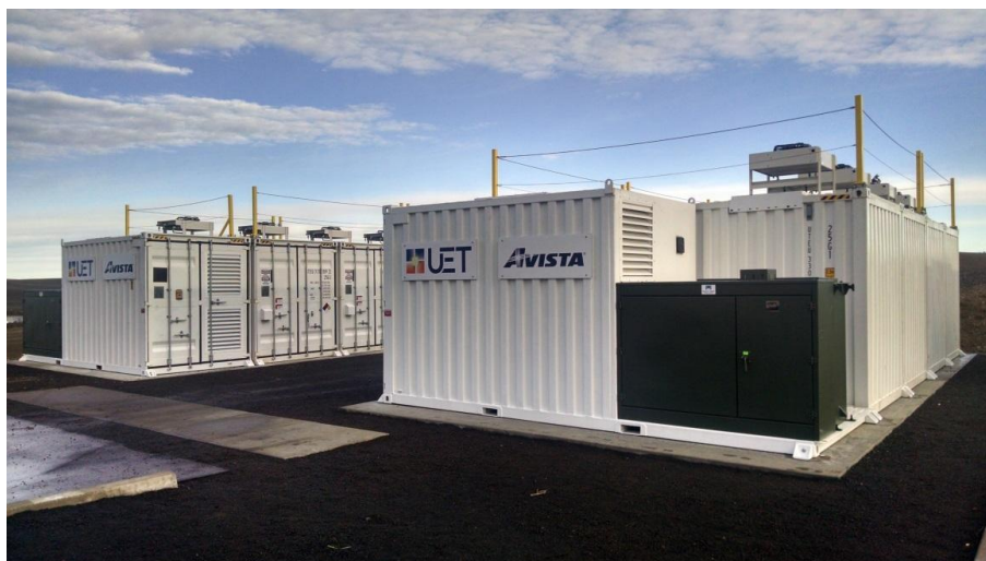
Turner Energy Storage Project, Pullman, WA
