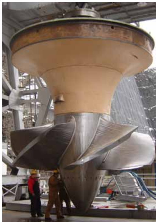
Noxon Rapids turbine upgrade
