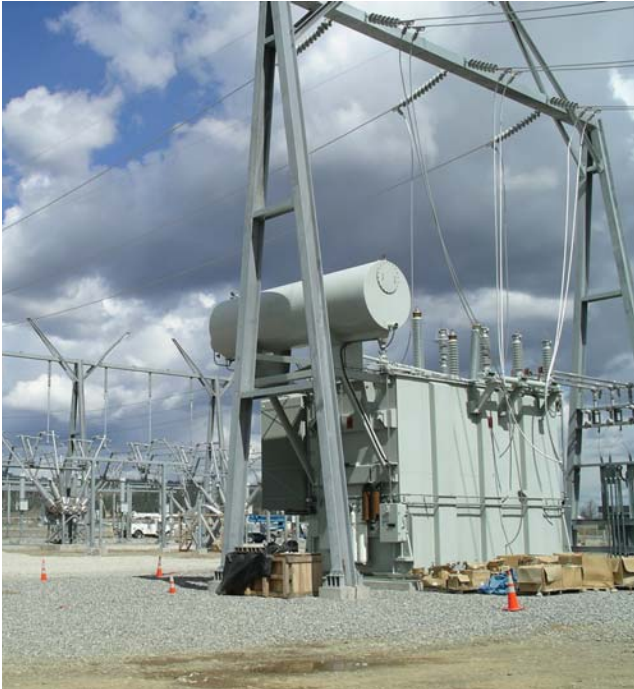
Transformer at Coyote Springs 2
