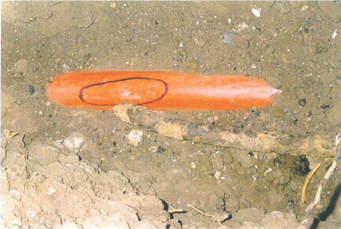
Figure 8 -- Brittle-like crack in pipe involved in August 1997 accident in Lake Dallas, Texas. The crack extends from the left to upper right of the area defined by the ellipse.
