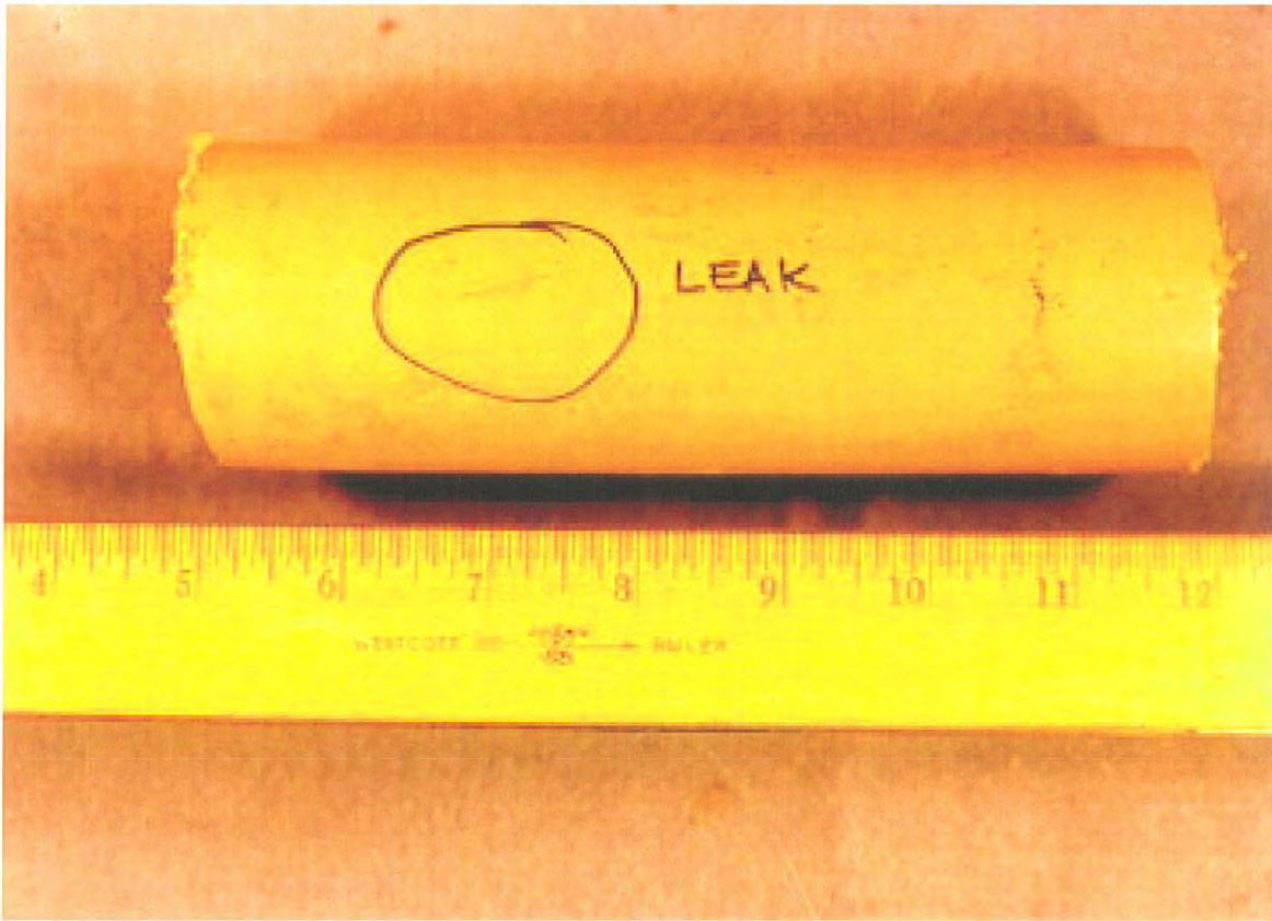
Figure 6 -- Slit fracture on a polyethylene pipe manufactured by DuPont that was found leaking and removed from a gas piping system.
