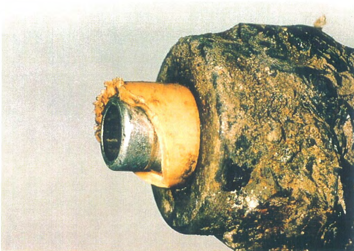
Figure 10 -- Close-up view of failed plastic pipe connection to steel tapping tee from site of Waterloo, Iowa, accident. A portion of the fractured plastic service line (light-colored material) remains attached to the tee.
