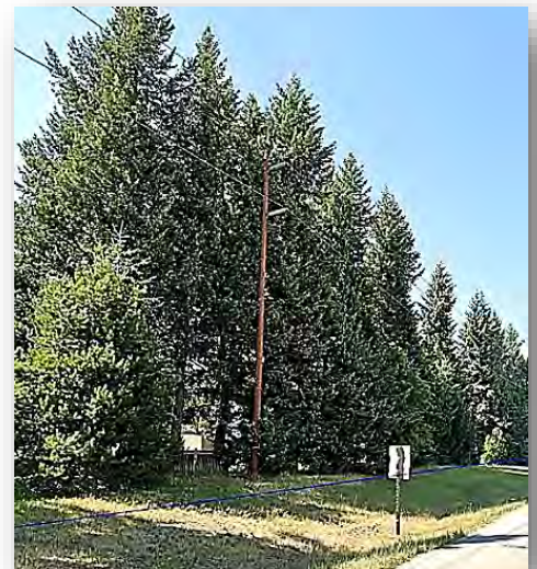
CDA-Rathdrum 115 kV along US Hwy 95
