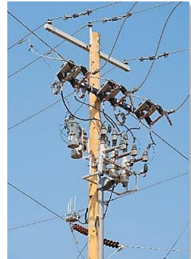
Figure 20. Dry Land Mode Device: Viper Recloser
