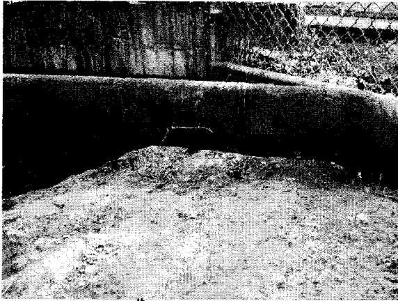
Figure 1. NE 11 th Avenue and NE Division water crossing, Camas, Washington: Pipe after concrete supports were removed.
