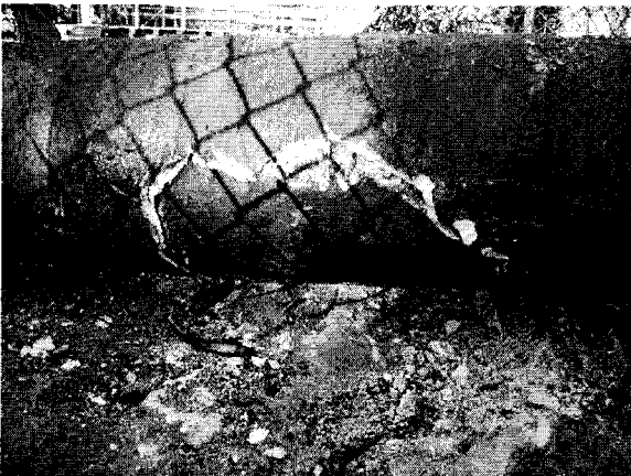
Figure 2. NE 11 th Avenue and NE Division water crossing, Camas, Washington: Close-up view of pipe condition after concrete supports were removed.
