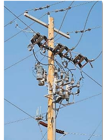
Figure 20. Dry Land Mode Device: Viper Recloser
