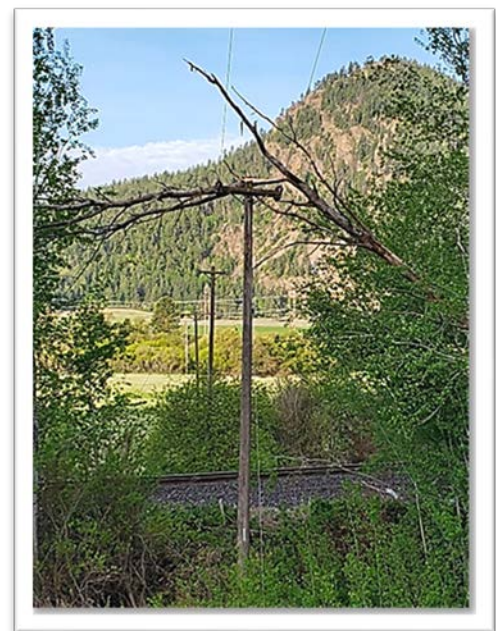
Figure 16. Dead tree falls into powerline
