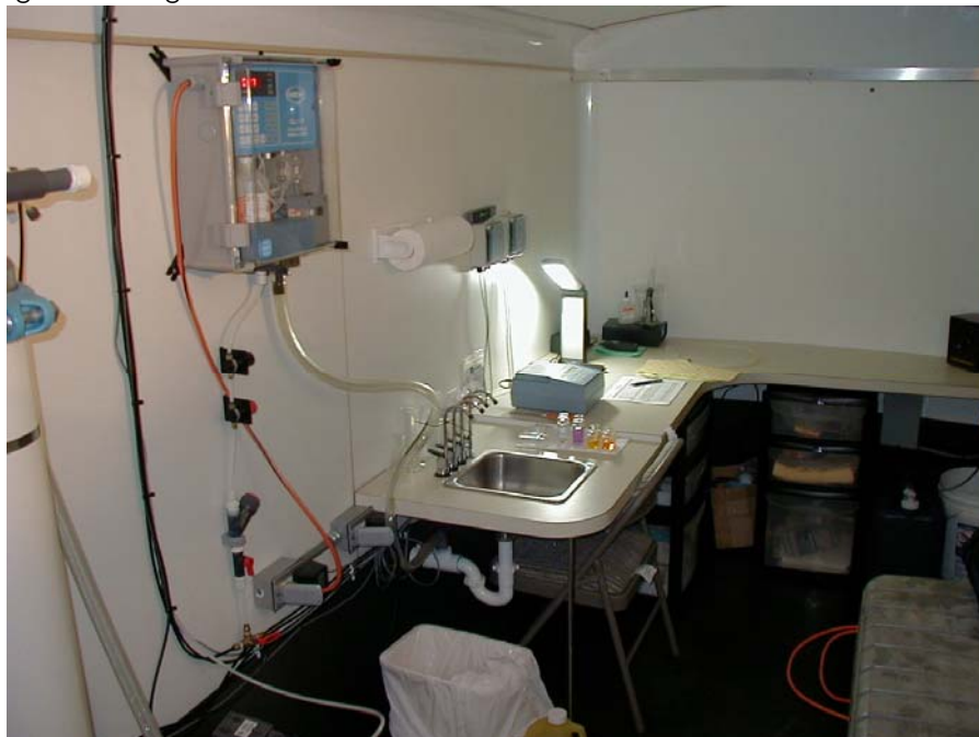
The front one-half of the trailer is shown above. The instrument foreground on the wall is an in-line chlorine analyzer. The smaller boxes on the wall above the light are electronic flow meters used to monitor cumulative as well as instantaneous flow for each treatment train in the pilot plant.
