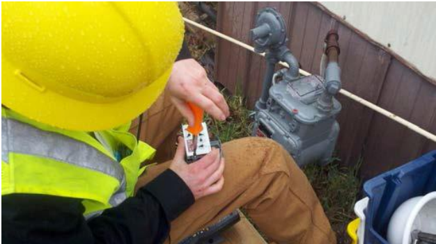
Retrofitting Natural Gas Meter Index with ERT
