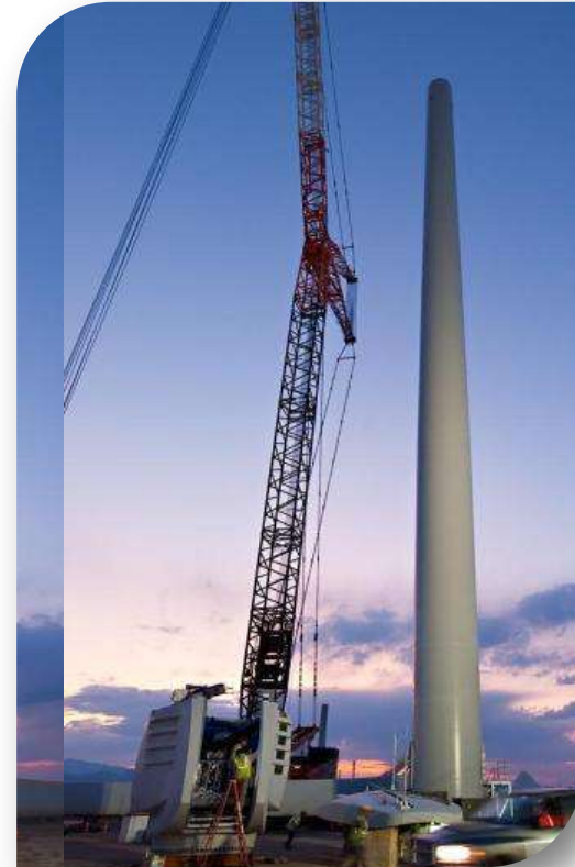
Milford Wind – 306 MW in Utah
