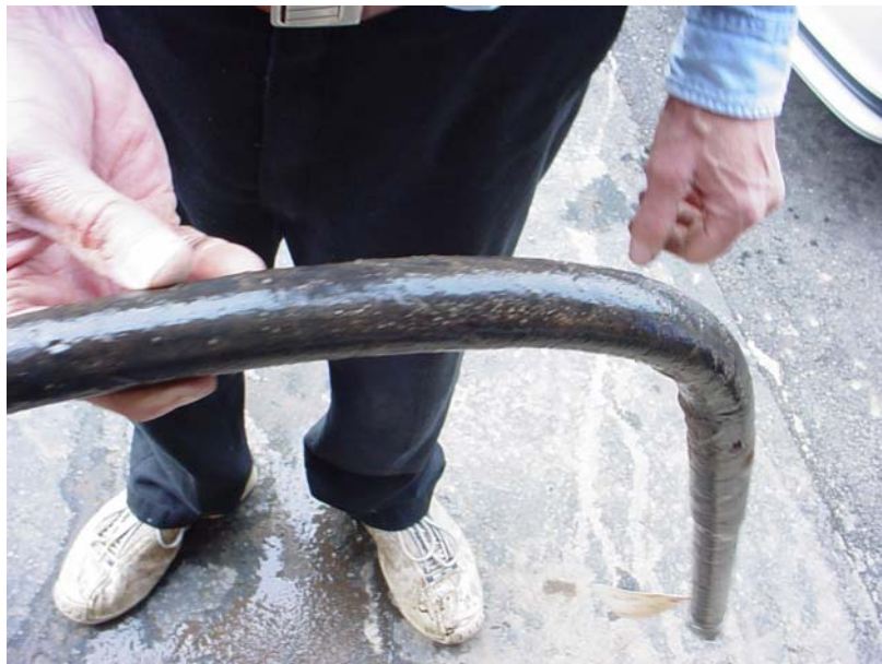
Photo 4: Example of bent coal tar service riser from Spiritridge with no visible coating holidays
