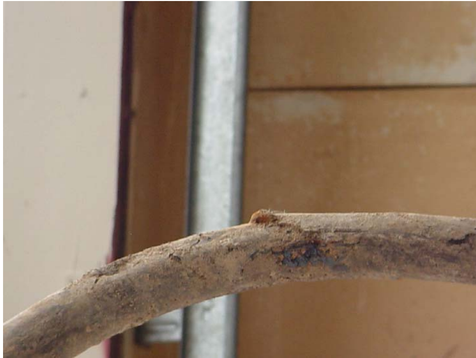
Photo 3: Examples of coal tar coated and bent service risers from Spiritridge subdivision with visible coating holidays
