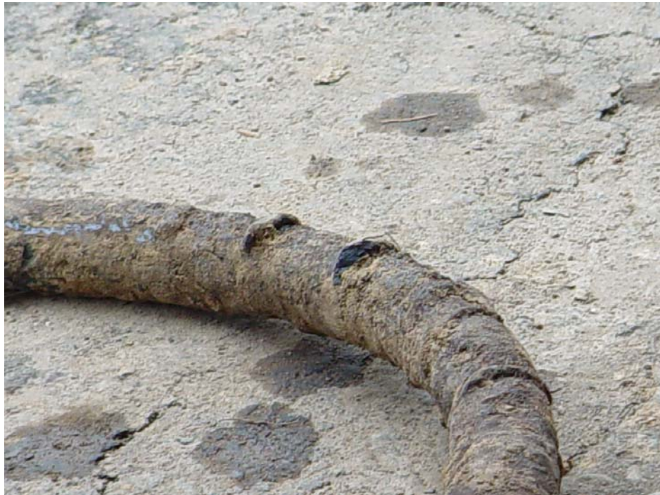
Photo 3: Examples of coal tar coated and bent service risers from Spiritridge subdivision with visible coating holidays
