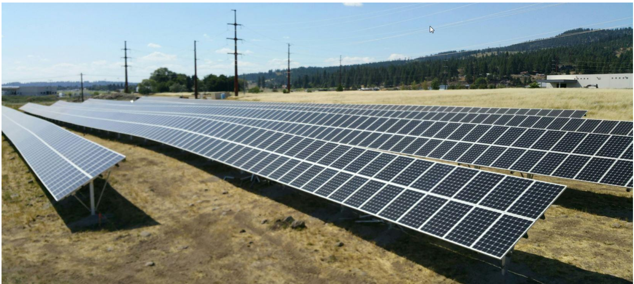
Boulder Park Community Solar Project
