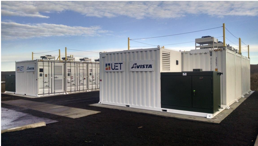
Turner Energy Storage Project, Pullman, WA
