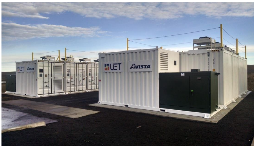
Turner Energy Storage Project, Pullman, WA
