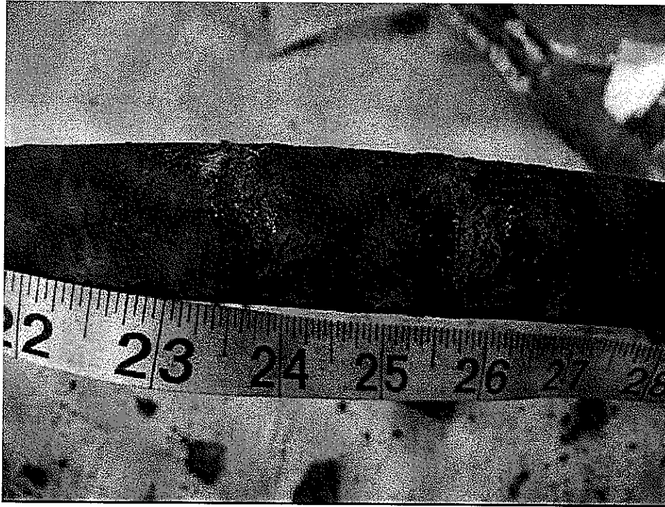
Figure 9. Photograph showing corrosion product after the coating was removed located between 23 and 26" from the upstream end of the pipe.
