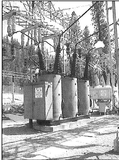
Sunset Substation - 115 kV Oil Circuit Breaker A-198 HV Breaker - oldest breaker on Avista's system.
