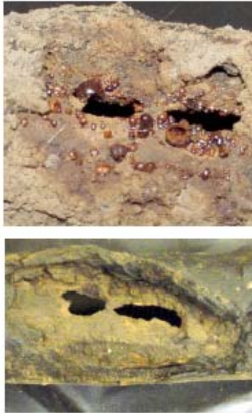
Figure 14. The leak site in Segment 10. Top photo – as received condition with protective plastic enclosure removed; bottom photo – debris and surface deposits removed.
