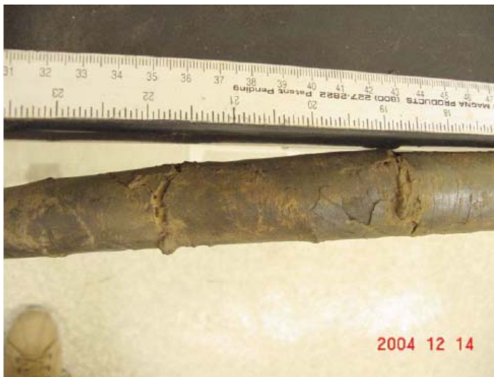
Item 2: Photograph from page 47 (Figure 34) of the CCTL Report, showing cracks in coating on extrados of pipe segment 10 not reported in Table 2 of the CCTL Report.
