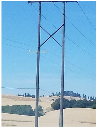
Latah-Moscow 115 kV Line, Built in 1924
