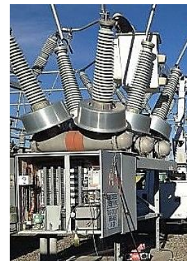
Avista High Voltage Circuit Breaker Undergoing Maintenance
