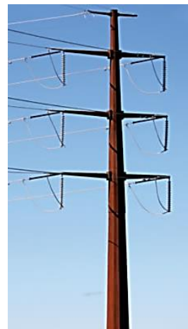
Above: Steel Self-Supporting Pole with Davit Arms
