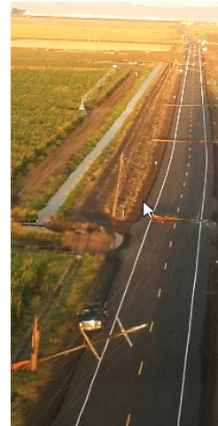
Right: Double Circuit Transmission Line (with ground wire on the top cross arms)
