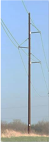
Above: Single Circuit Transmission Lines with the traditional three phase conductor
