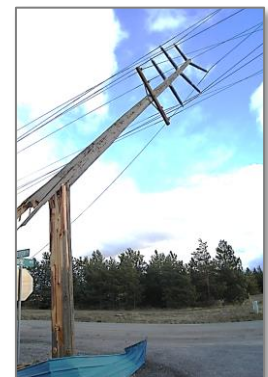
A big windstorm in Rathdrum snapped several transmission poles in the area in 2014
