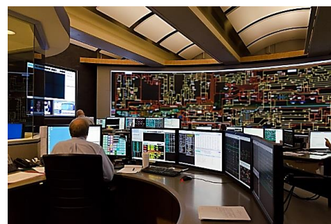
Typical Utility Dispatch Center
