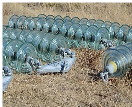
Strings of transmission insulators, sometimes called bells
