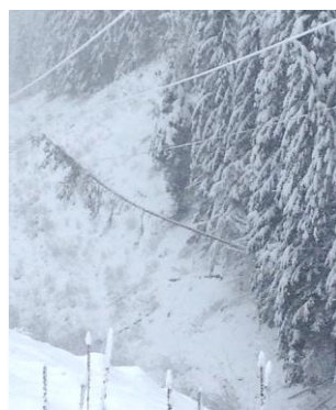
Left: Tree caused outage on the Cabinet-Rathdrum line
