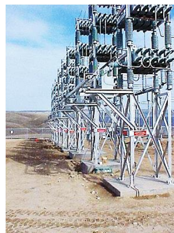
Dry Creek Capacitor Bank
