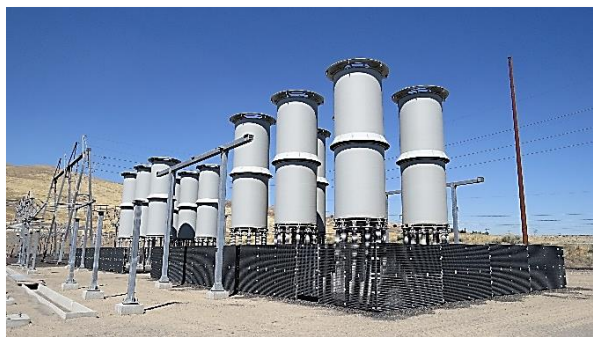
North Lewiston Reactors help regulate the voltage and reactive power in this area
