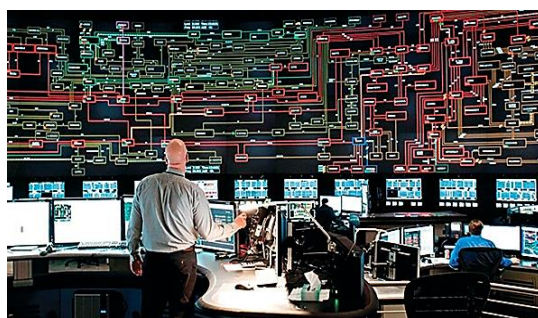
Utility Control Center
