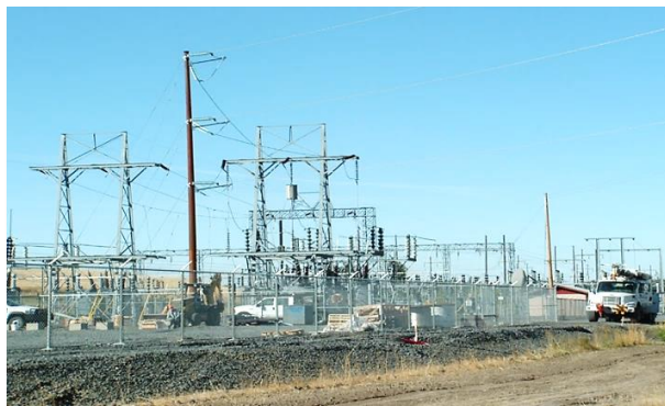
Typical Avista Transmission Substation
