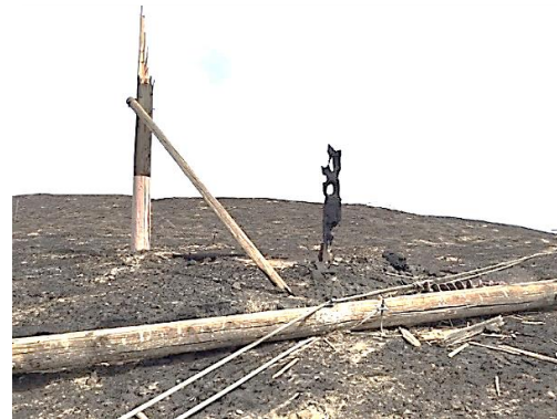
The Company has experienced the success of this coating in several recent wildfires. Fire burned through the Walla Walla – Wanapum 230 kV line in 2017. As you can see, the fire retardant portion of the pole is safe. Unfortunately this fire burned high enough due to winds that it reached above the protected level.
