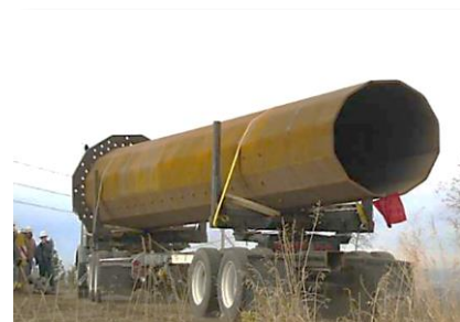
The 50 year old Beacon-Rathdrum line was rebuilt as part of the West of Hatwai Project
