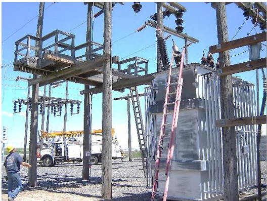
Transformers in Nez Perce Substation
