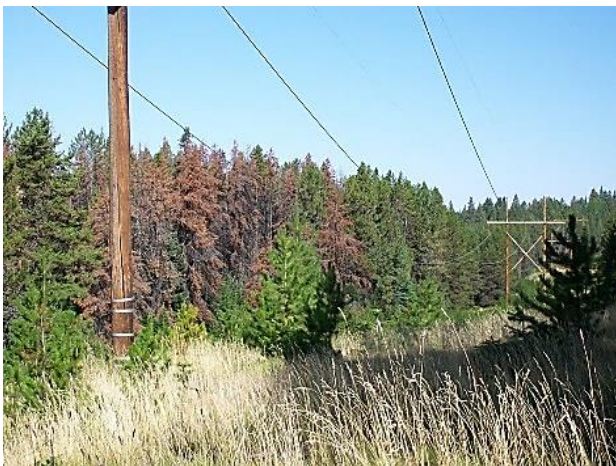
Western pine beetle infestation in Lodge Pole Pines on the Lolo Oxbow 230 kV line
