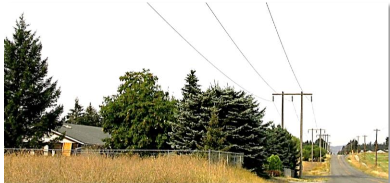
Roadside 115 kV transmission line. Requires aerial lift truck and chipper crew every 3 years to maintain clearance.
