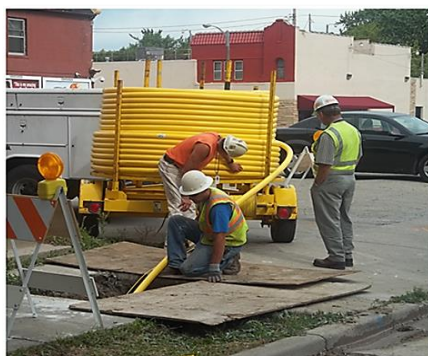
New main pipe be installed in the borehole created by the horizontal drilling
