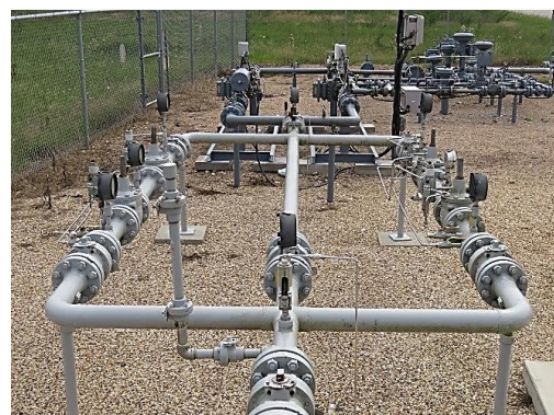
Natural Gas Regulator Station
