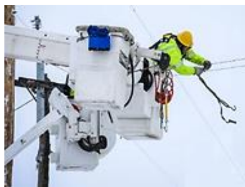
Lineman in Davenport restoring service in a snowstorm. Courtesy of Infinity Rose Photography
