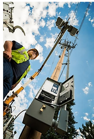
Adding Grid Modernization Technology to a Feeder
