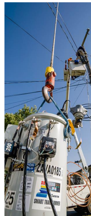
Avista “Smart” Transformer
