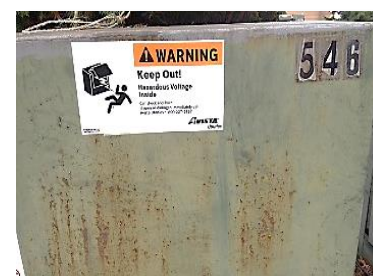
Below: Paint failure can lead to rust-through of cover
