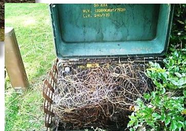
Below: Vines Growing Inside a Transformer Box
