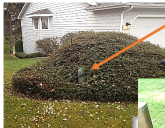
Left: Transformer Covered by Shrubbery
