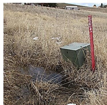
Underground equipment now in a bog
