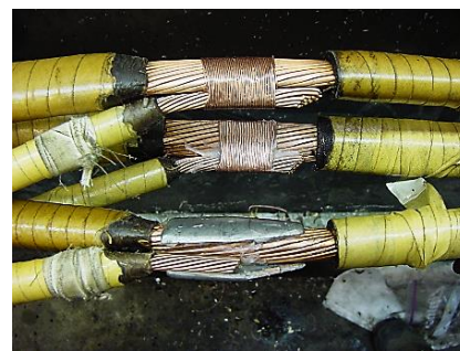
Downtown network crew beginning the process of filling cable with lead to create a solid splice; this type of work is considered an art
