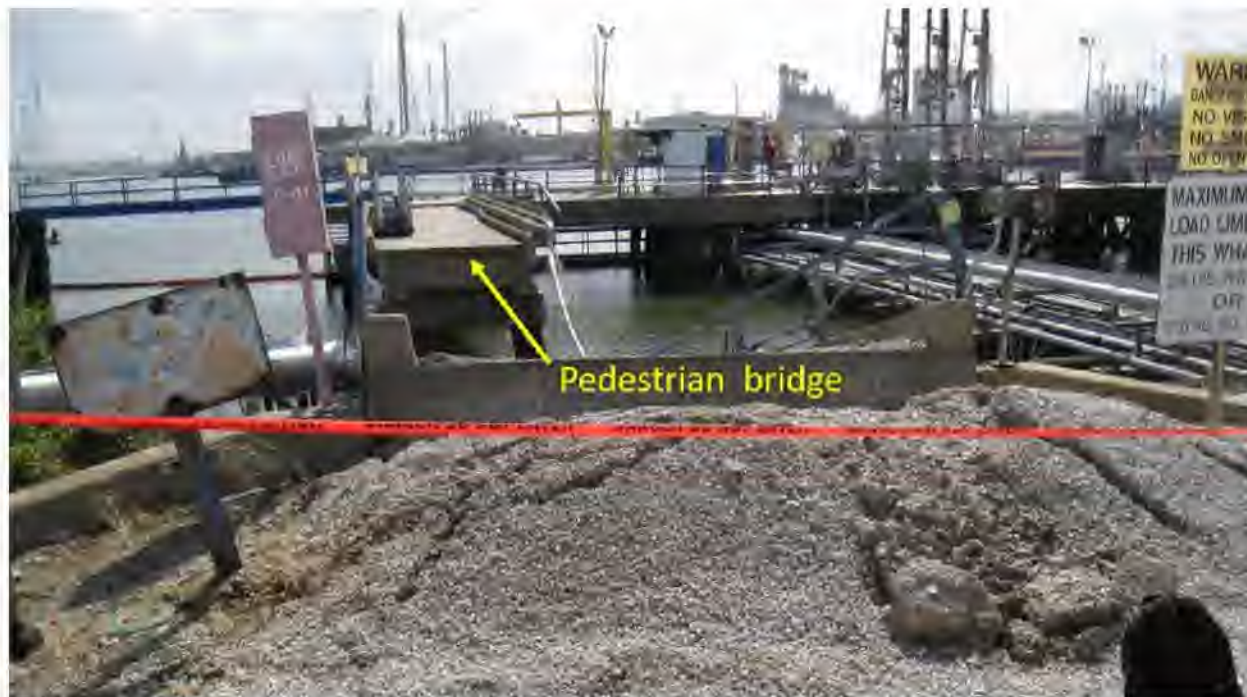
TPC facility on Houston Ship Channel. The impact pushed the pedestrian bridge off its support, crushing conduit below. (Photo by Coast Guard)
