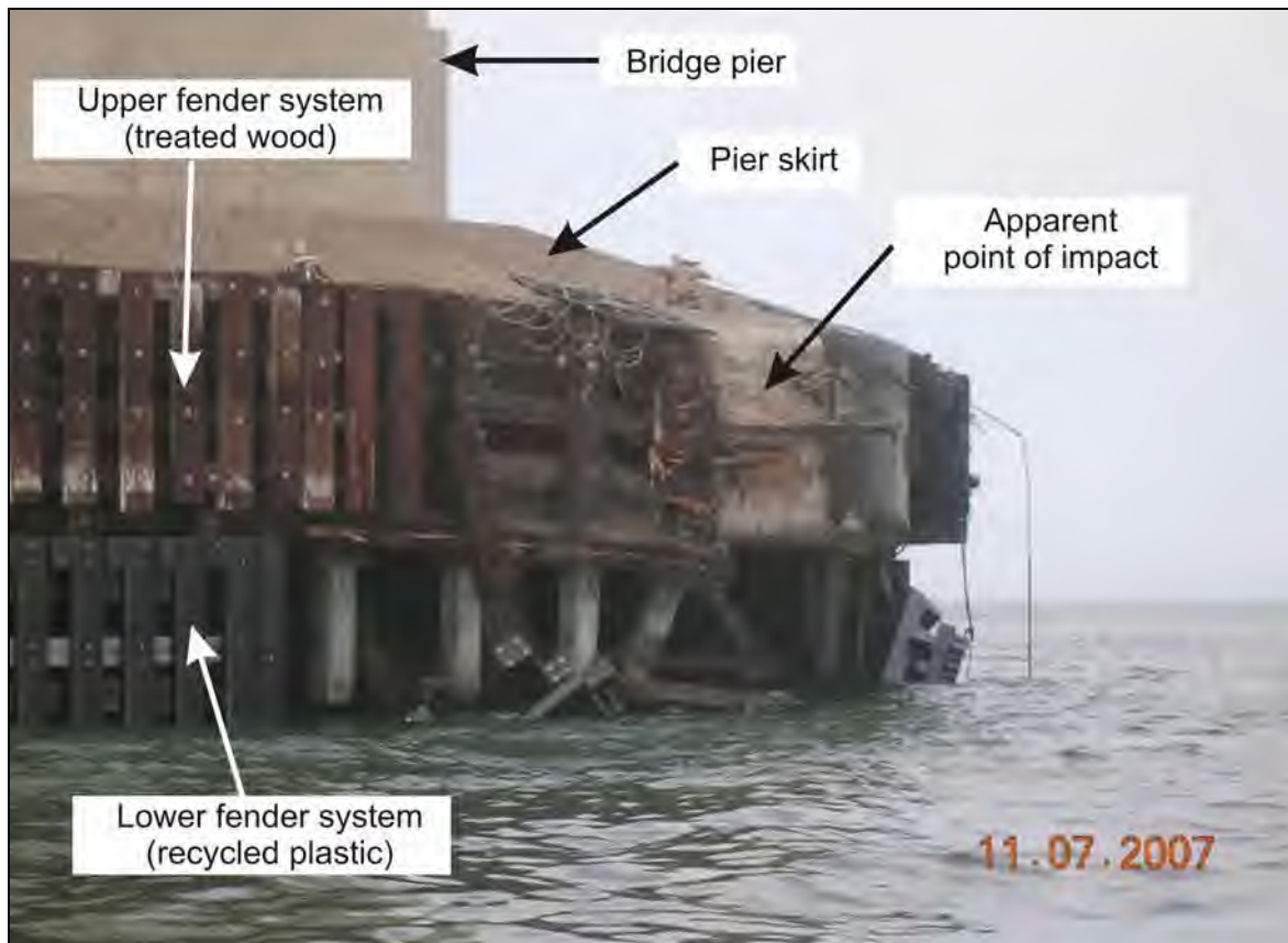
Figure 6. Close-up view of the fendering system at the base of the Delta tower showing the likely point of impact and a portion of the 100-foot-long damage area.
