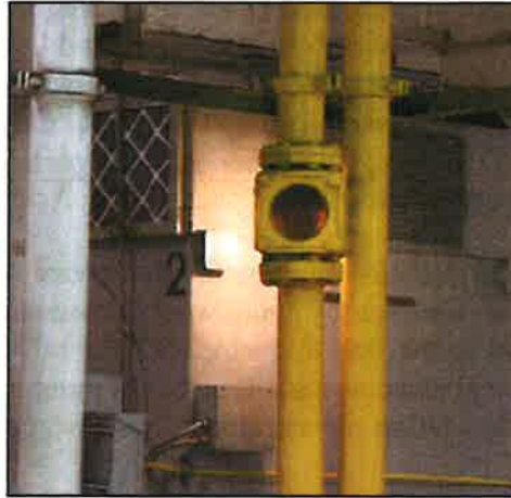
Figure 12. Bull's-eye for monitoring lube oil flow from gravity tank. (Photo from El Yunque )
