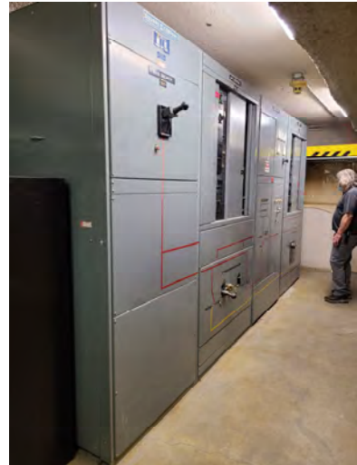
Existing 208/120V Main Switchboard located in basement
