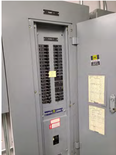
Existing age of Panelboards in Building
