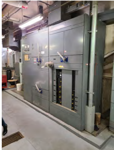
Existing Main 480/277V 3,000 A Switchboard
