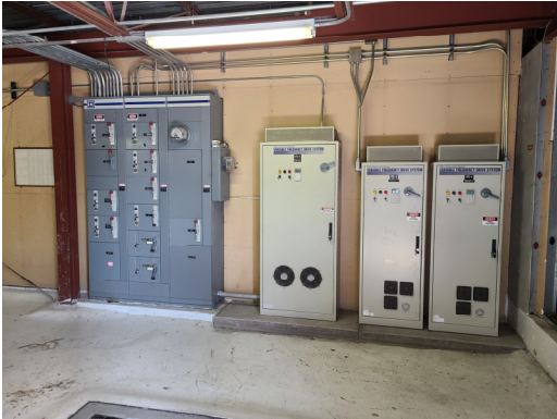
Existing MV Equipment
