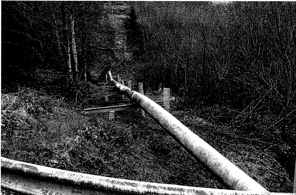
The aboveground section of the K-B Pipeline on pile supports looking toward the active landslide area at the top of the slope.
